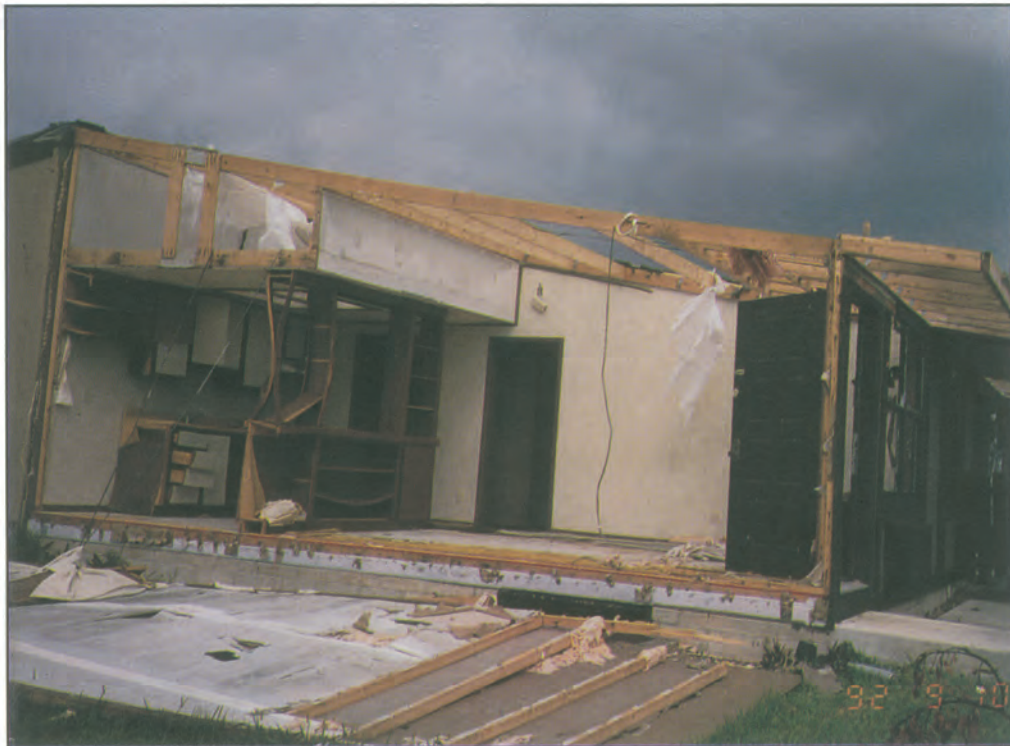
FIGURE 19. Modular home. End wall of end unit separated from unit; withdrawal of nails along eave line and roof sheathing failure were also observed.
